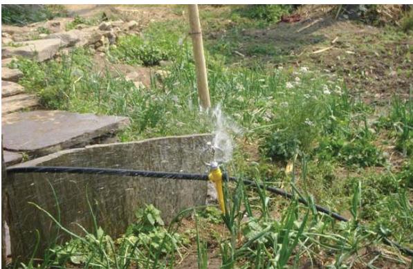
Sprinkler system connected to drinking water tap as a part of multiple water use system
